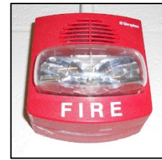
Fire Alarm Strobe Light
