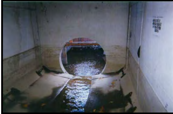
CSO STORAGE TANK OUTLET
