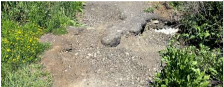
Washout at pond outlet
