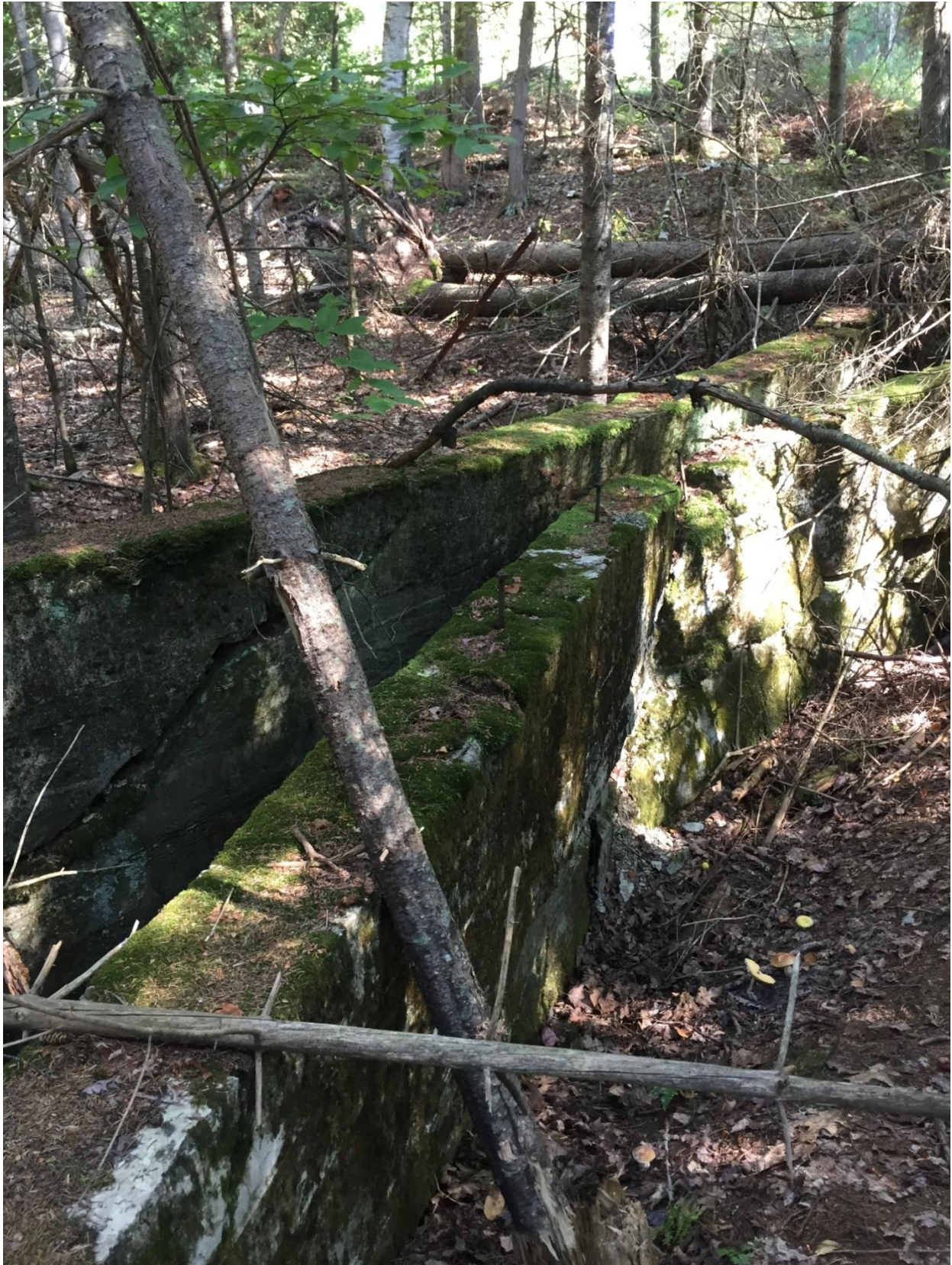
Photograph 4: The front edge of the concrete structure that accommodated targets has collapsed onto the back edge.
